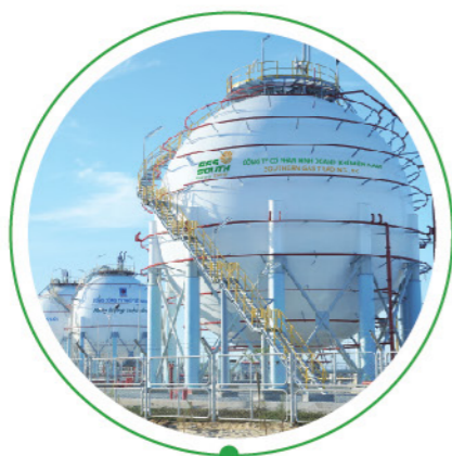
Dung Quat LPG warehouse in Quang Ngai (1,500 tons), taking directly from Dung Quat Oil Refinery, supplying LPG to the Central region
