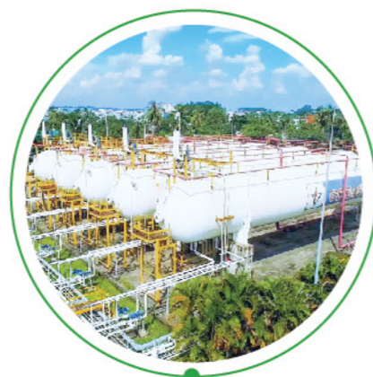
VT GAS LPG warehouse in Dong Nai (1,000 tons)
